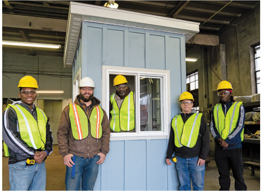
Build Ready students construct a guard shack at training partner SUNY EOC's campus.
