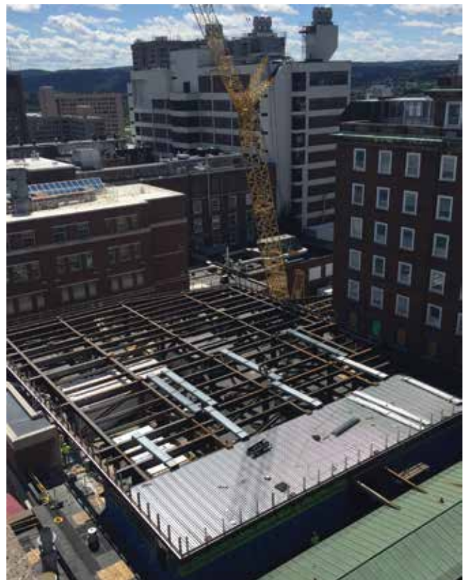
An aerial view of the new 52,000-square-foot emergency department now under construction at Crouse Health.
